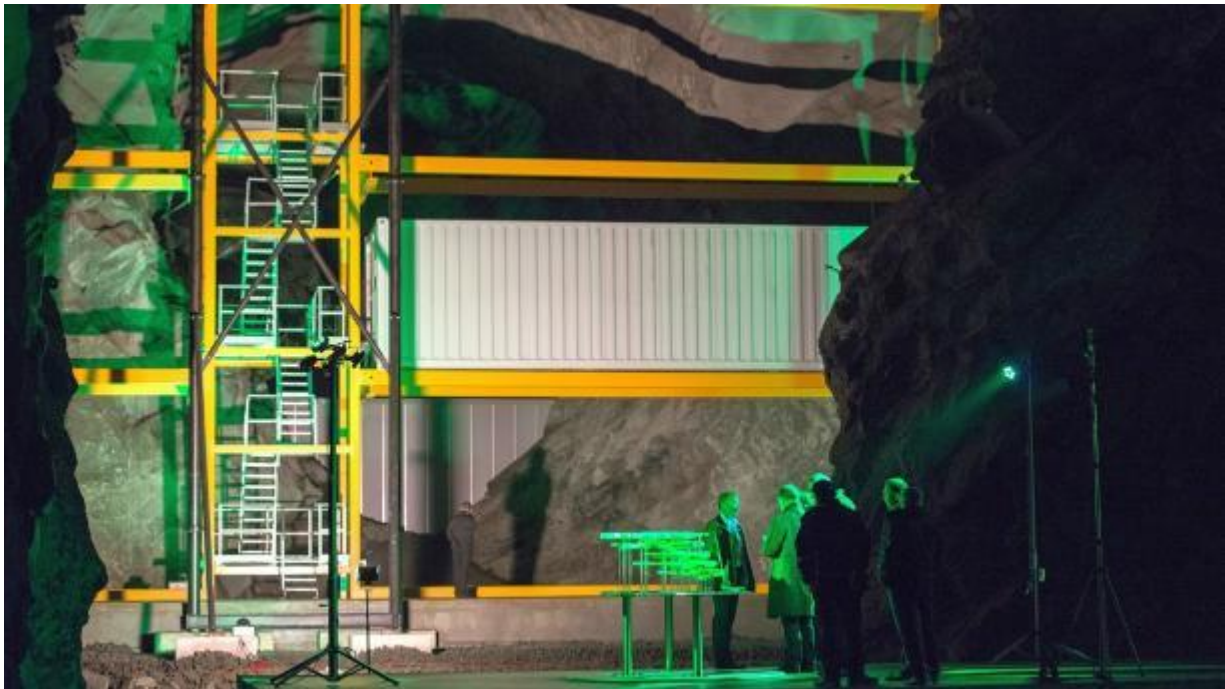
Blick ins Lefdal Mine Datacenter
